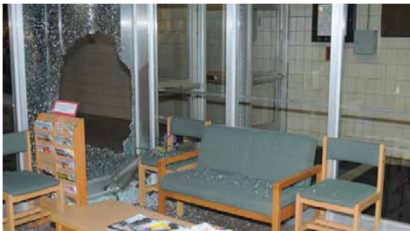
Figure 31. Window with shattered glass, supposedly blown out by “the shooter,” next to the front lobby doors (2013 final report, Walkley scene photos).
