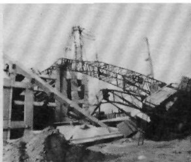
ABOVE: October 23, 1986, the luckiest day of my life. During construction of a 2,700-car garage at the Trump Plaza Hotel and Casino in Atlantic City, the boom of a huge crane reached out too far to pick up a 22-ton beam; the crane toppled over, and a large section of the garage collapsed. Minutes before the accident, at least a hundred workers were on the site. The crew had just left for a coffee break, and no one was hurt.
